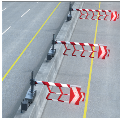
Tapered gates used to perform an automated lane closure
